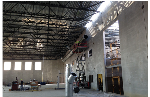
Overhead Ductwork in Student Activity Center
