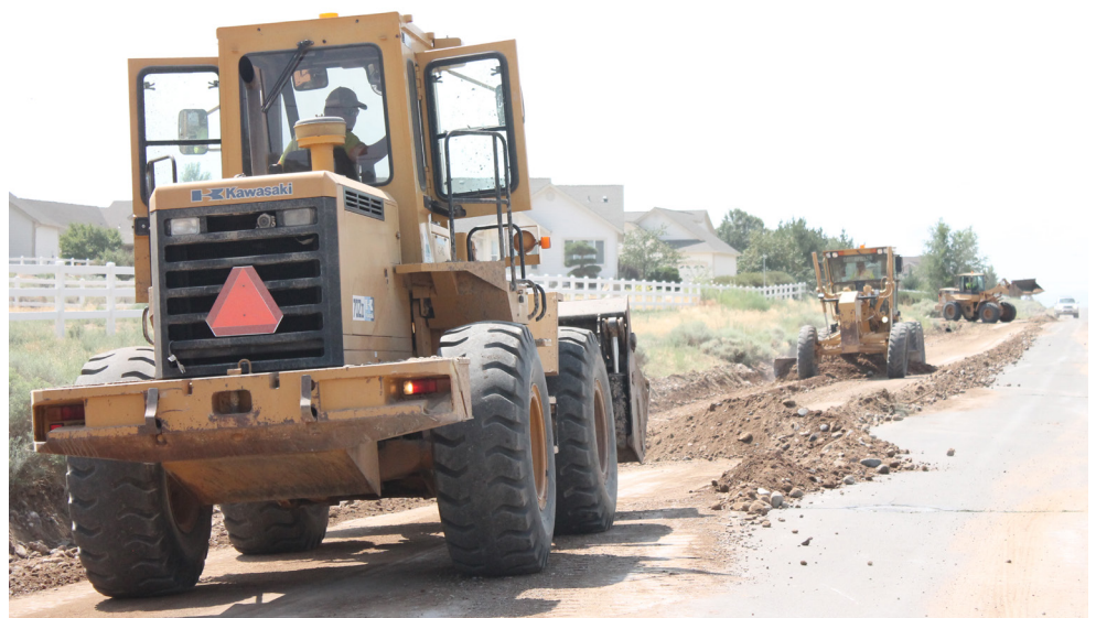
Douglas County Road Crews have made flood clean up a priority, cleaning streets and culverts daily.
