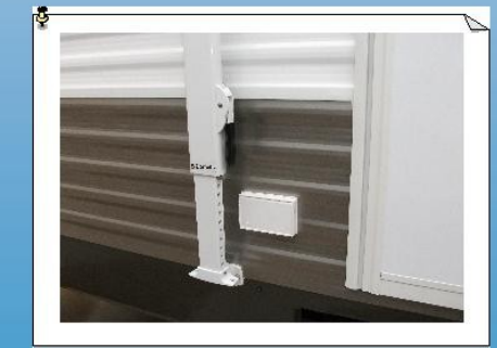
A dedicated outlet for awning lights is powered by an interior switch for convenience.
