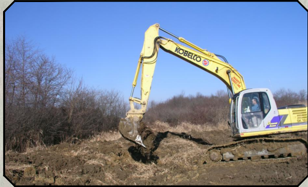
Construction occurred in fallow agricultural fields and involved creating small broad berms to disrupt surface flow and restore site hydrology. In addition to retarding surface water movement, a tile search was conducted to disrupt subsurface drainage of the site.
