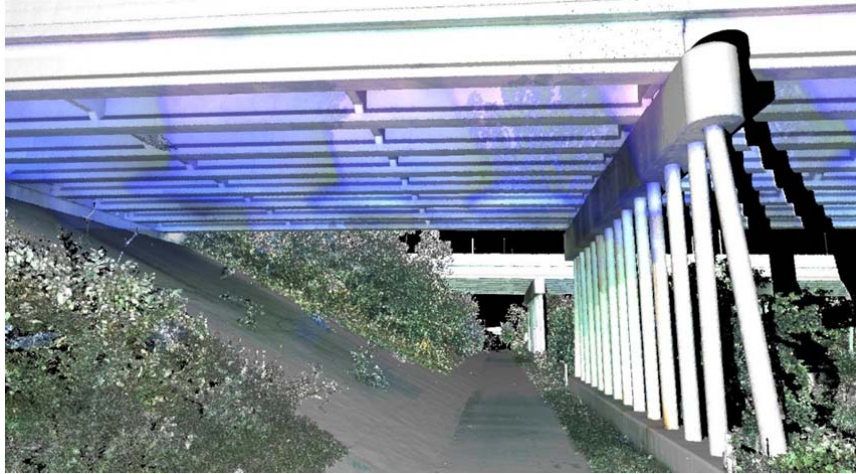
Point cloud rendering courtesy of Great Lake Geomatics. NB lanes of I-275, Lower Branch River Rouge, Canton Township, Michigan.
