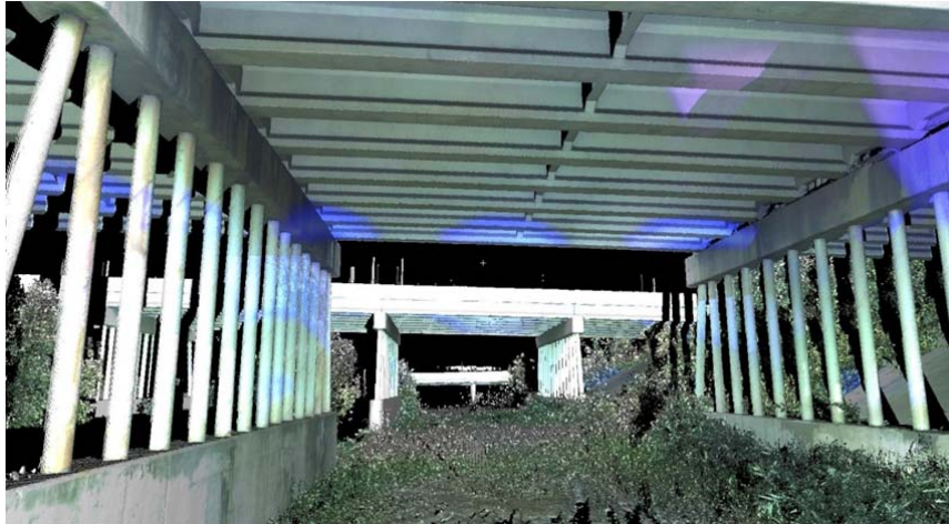
Point cloud rendering courtesy of Great Lake Geomatics. NB lanes of I-275, Lower Branch River Rouge, Canton Township, Michigan.
